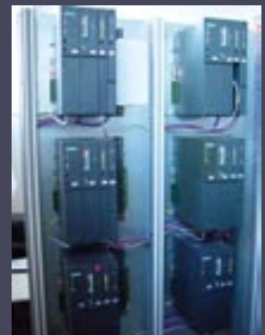
At the heart of the solution: Simatic PCS 7 controllers.
